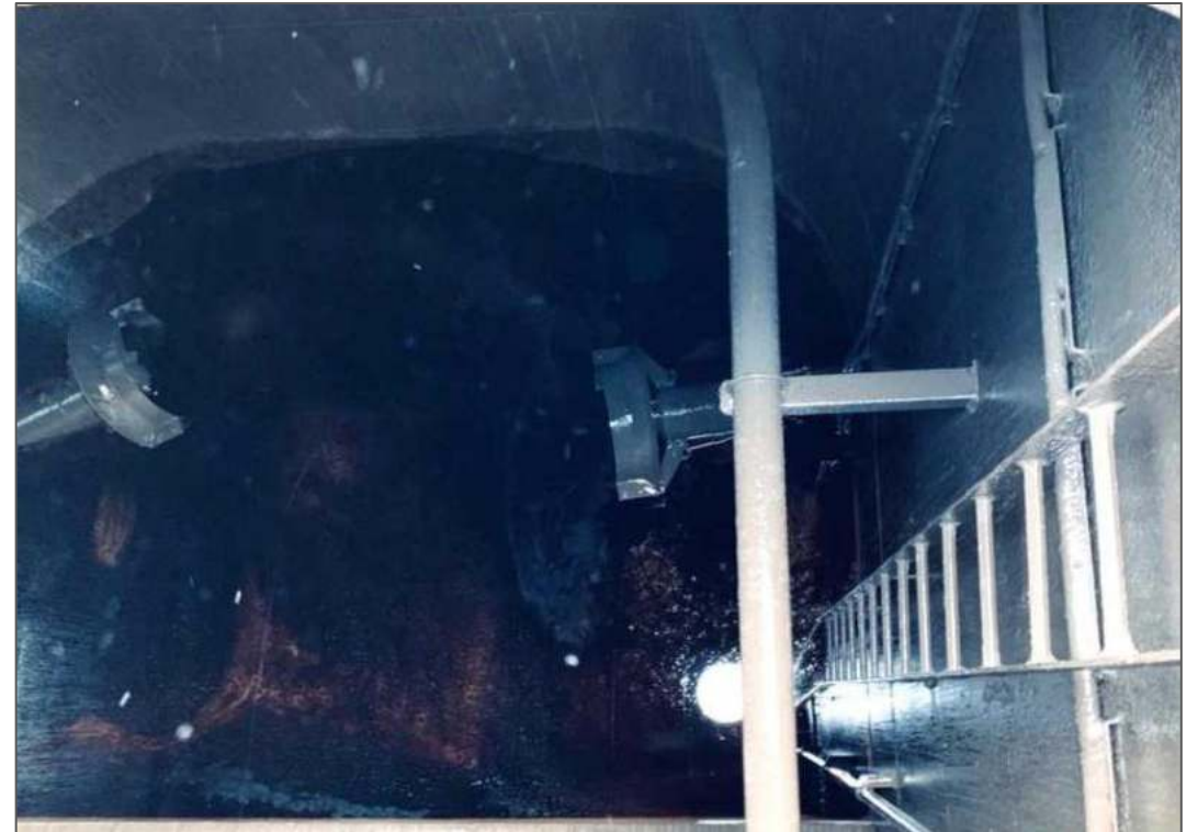
BASE OIL TANK
