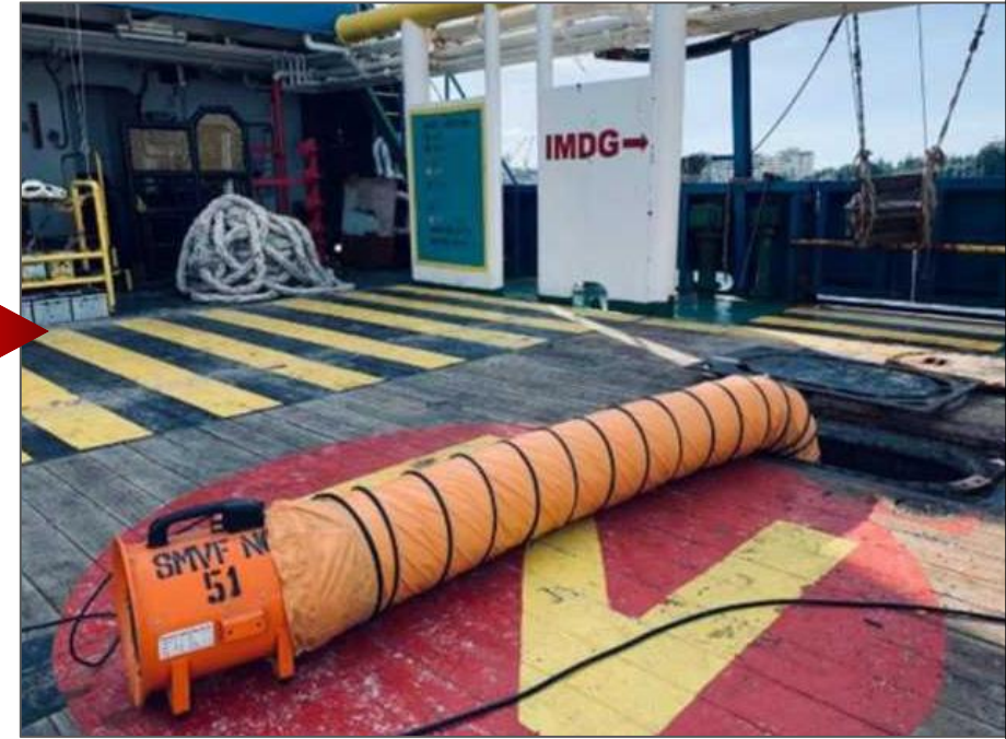
VENTILATION PROCESS CONDUCTED TO REMOVE TOXIC GAS
