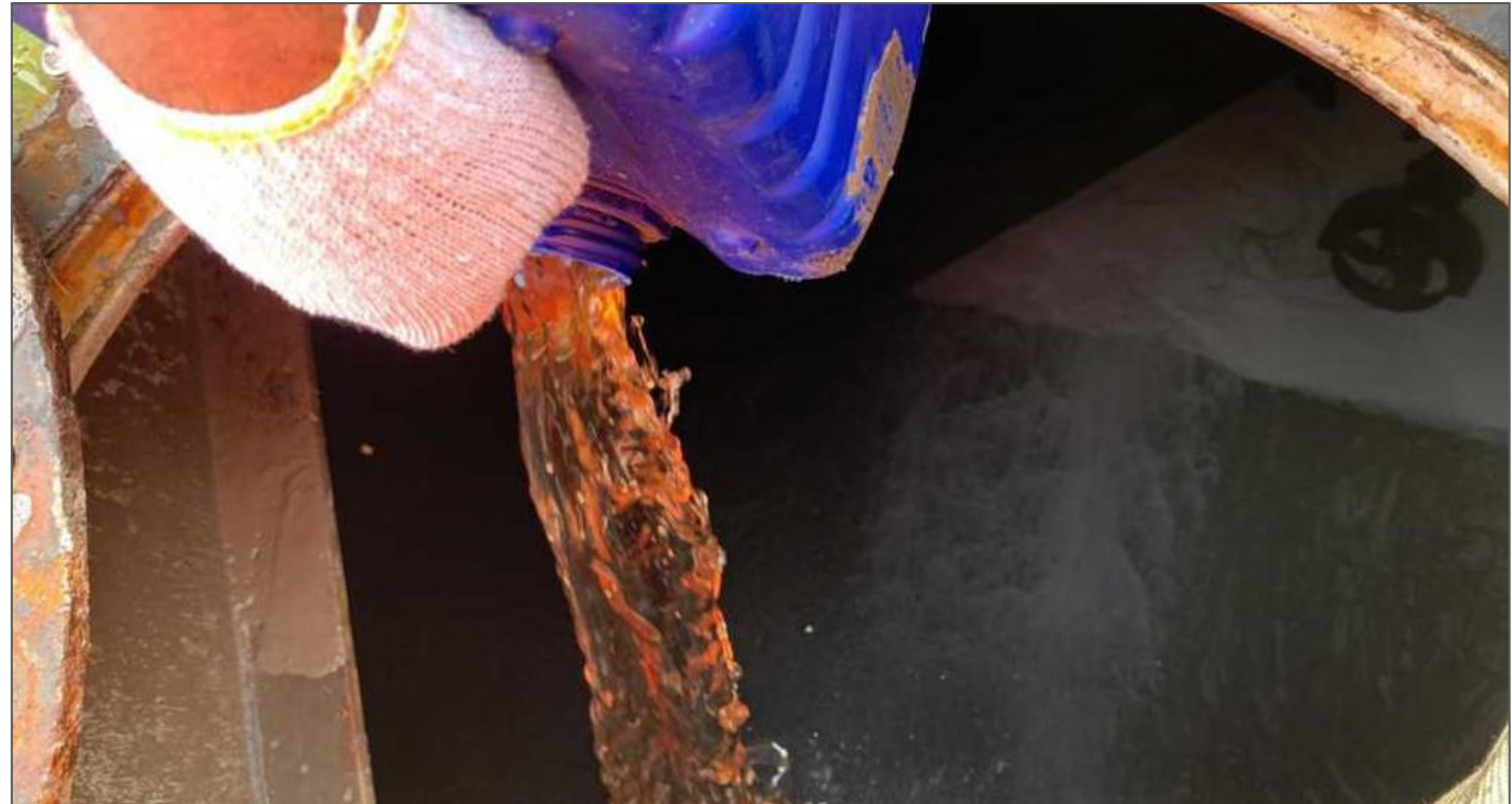
POUR IN CLEANING DEGREASER BEFORE FLUSH LINE ACTIVITY
